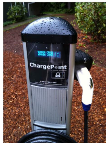
ChargePoint/Coulomb Level 2 Charging Station
